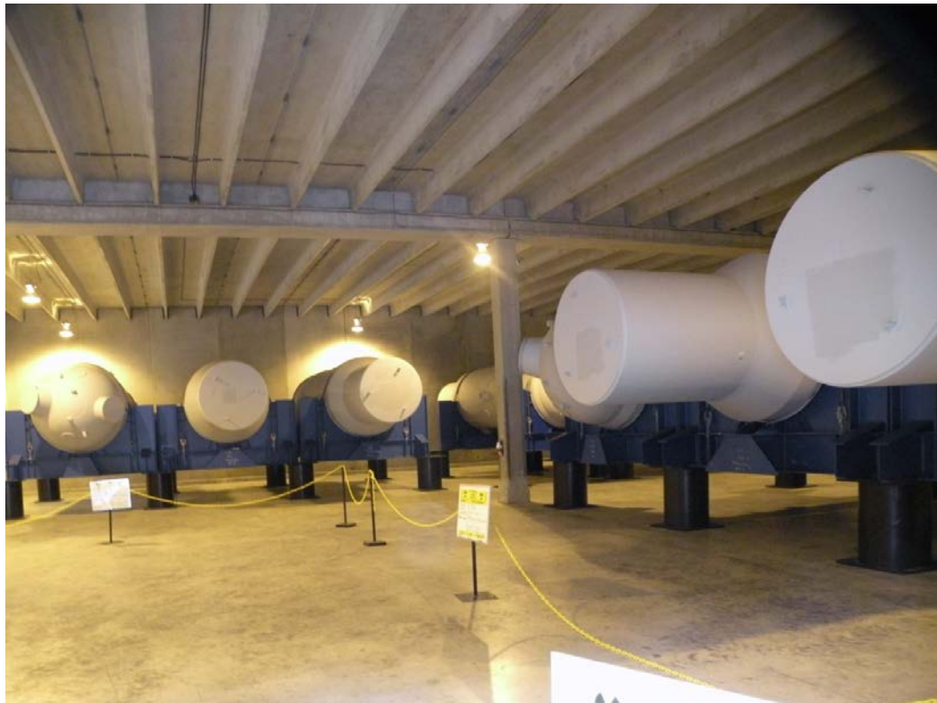
Figure 11: Storage of Steam Generators
